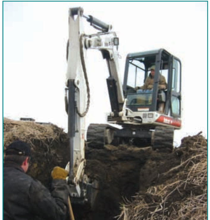
The cost of drainage water management includes installation, as well as purchase and management of the structure.
